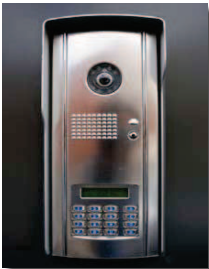
Access control panel on external doors.
